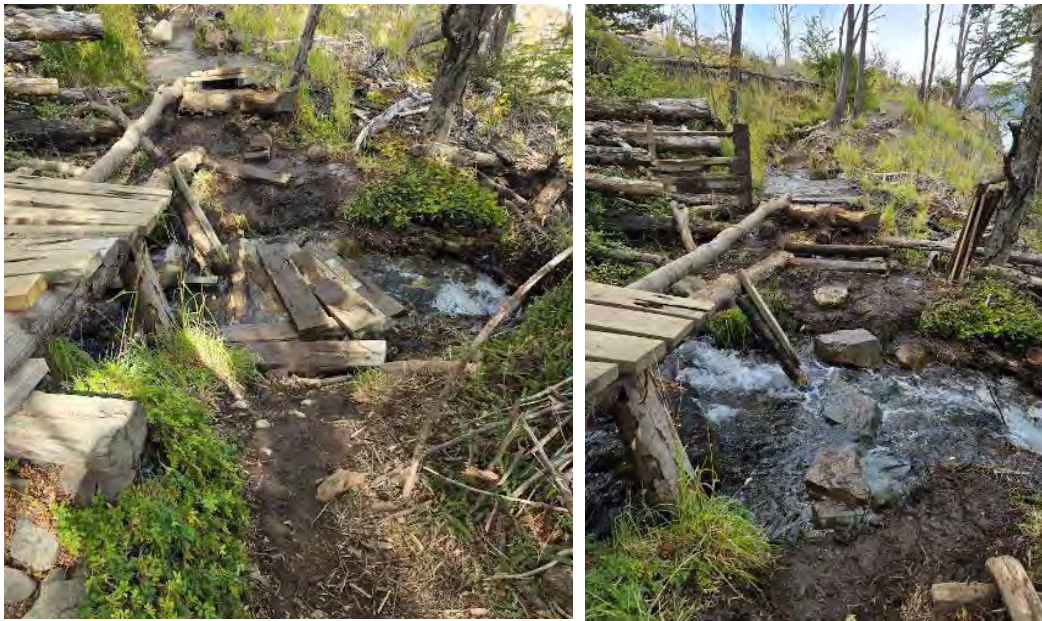
Before and After improving dangerous and slippery water crossing
