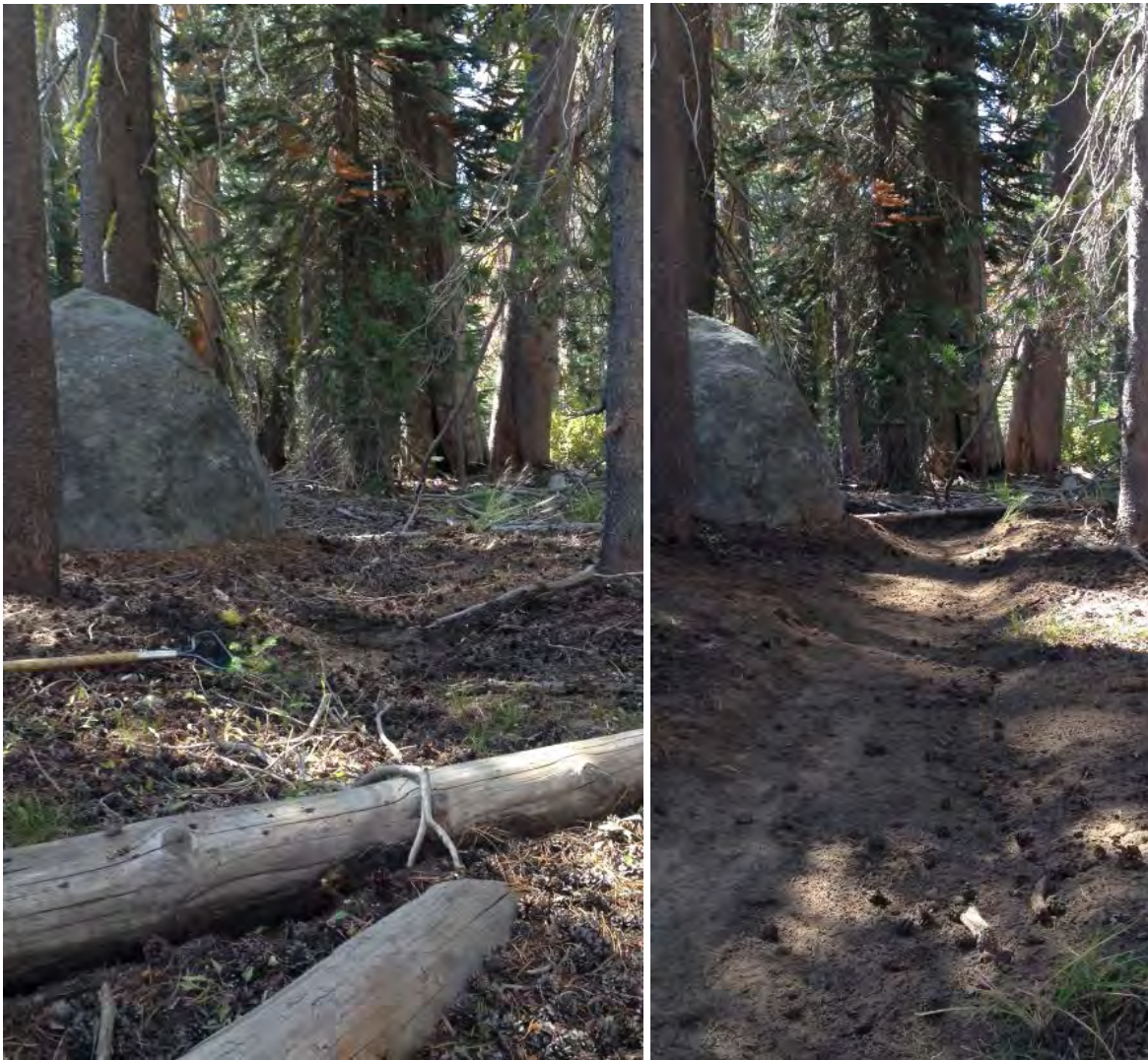
A before and after on one of the many drainages repaired by volunteers.
