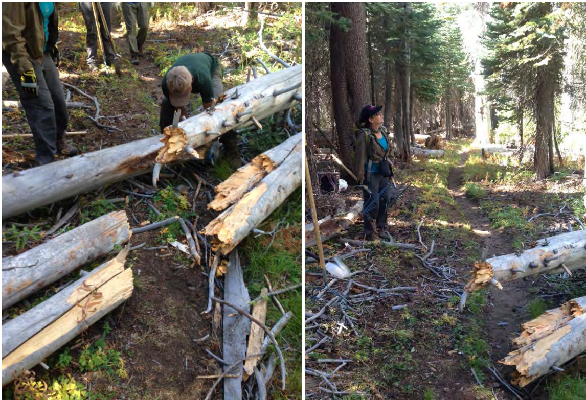
Before, the trail was covered by a downed tree that make the trail difficult to navigate.
