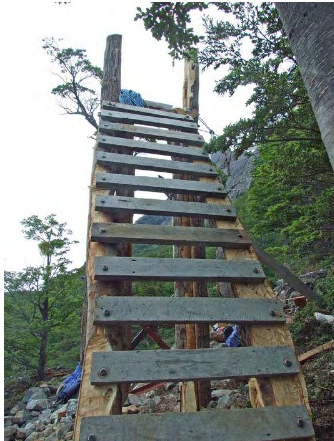
This is what the tall tower on the south side looked like after the steps for the ladder were attached to the diagonal supports
