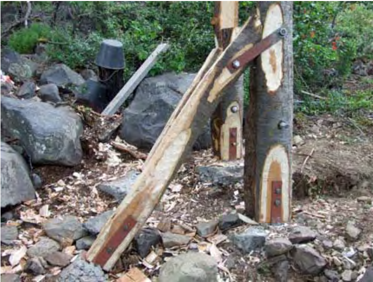
This is a side view of the short tower on the north side, just after the diagonal supports were attached
